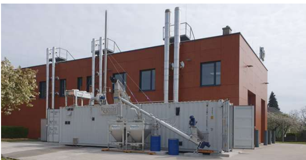
Pilot-plant in container on the Wieselburg site of BEST GmbH, Source: BEST GmbH
